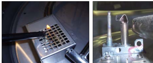
Fig. 2 Blow Out Box- Pilot Assembly Inside.
